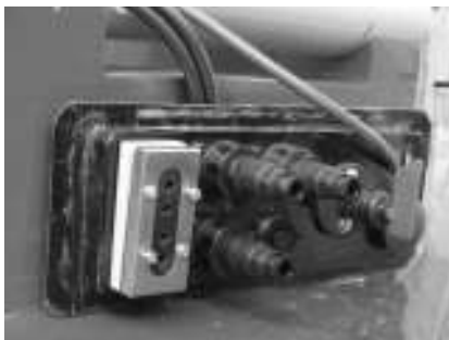
Figure 3a: One of the front panels showing the connectors, cable gland, isolator and an emergency switch
