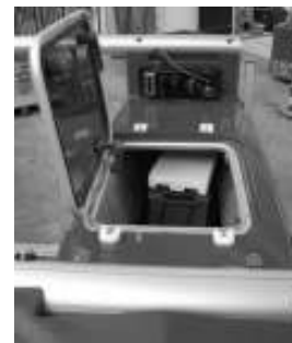
Figure 3b: Layout of components including batteries, hatch and front panel are shown on one of the hulls
